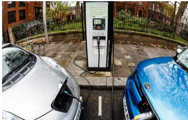
Electric vehicle charging points
