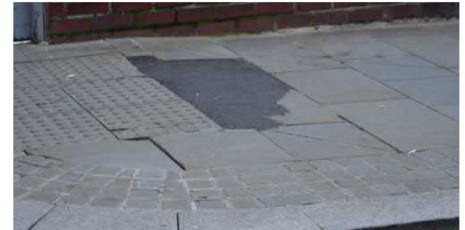
Natural stone paving scheme along Derby Street repaired with tarmac
